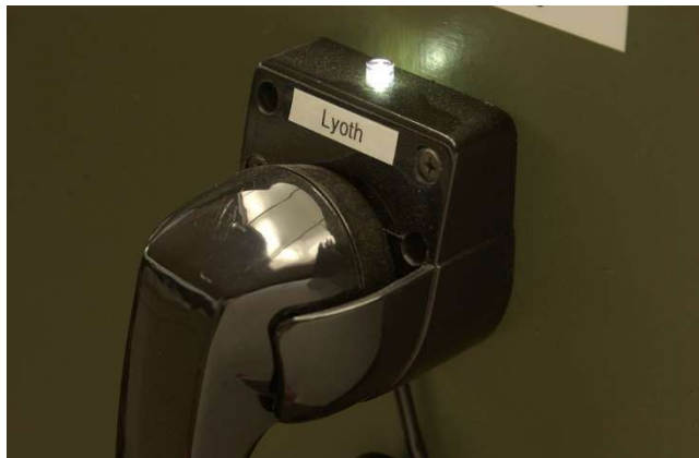
Figure 21 - LED installed on Cup Hook (courtesy of Tommy Holt)
